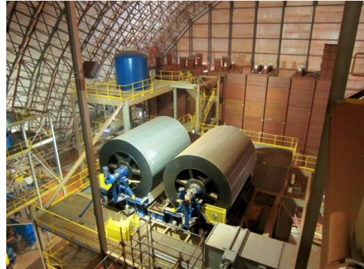
Processing equipment under covered dome plant structure
